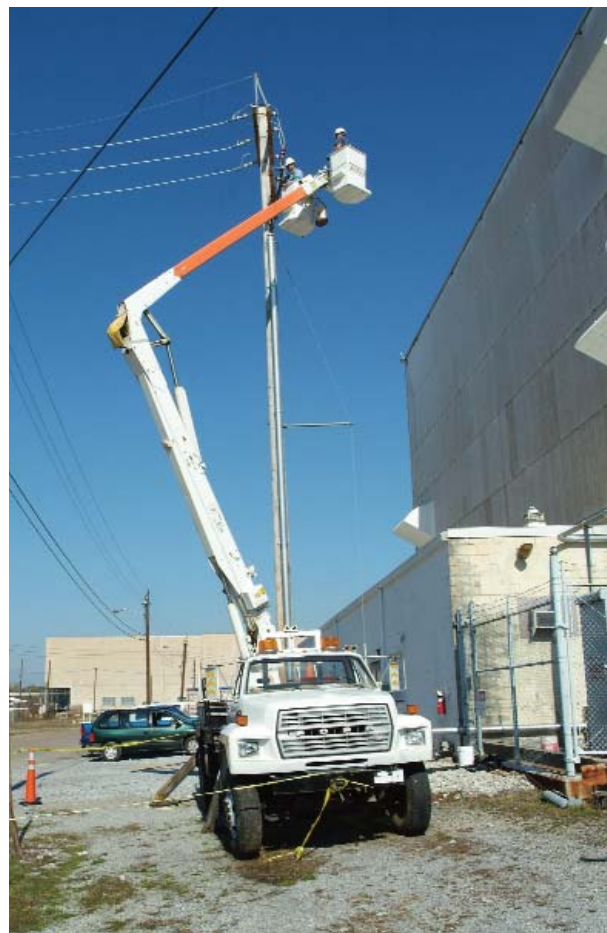
Overhead power lines are run to the area where a treatment system is to begin extracting TCE from beneath the surface and significantly reduce the site's largest source of off-site contamination.
